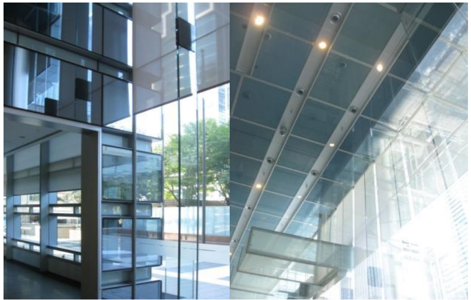
Tower B lobby where curtain wall "punches through" glass fin supported storefront.
